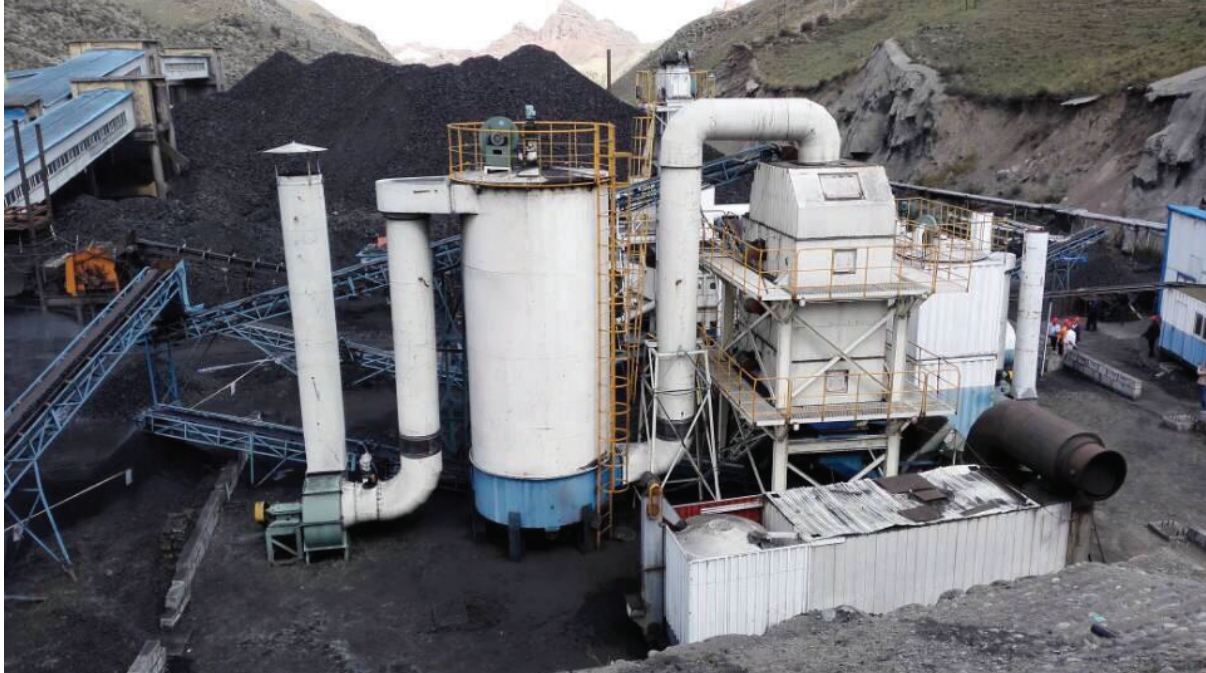
Figure 1: Dry Dense Medium plant in operation at Shenhua, China.
