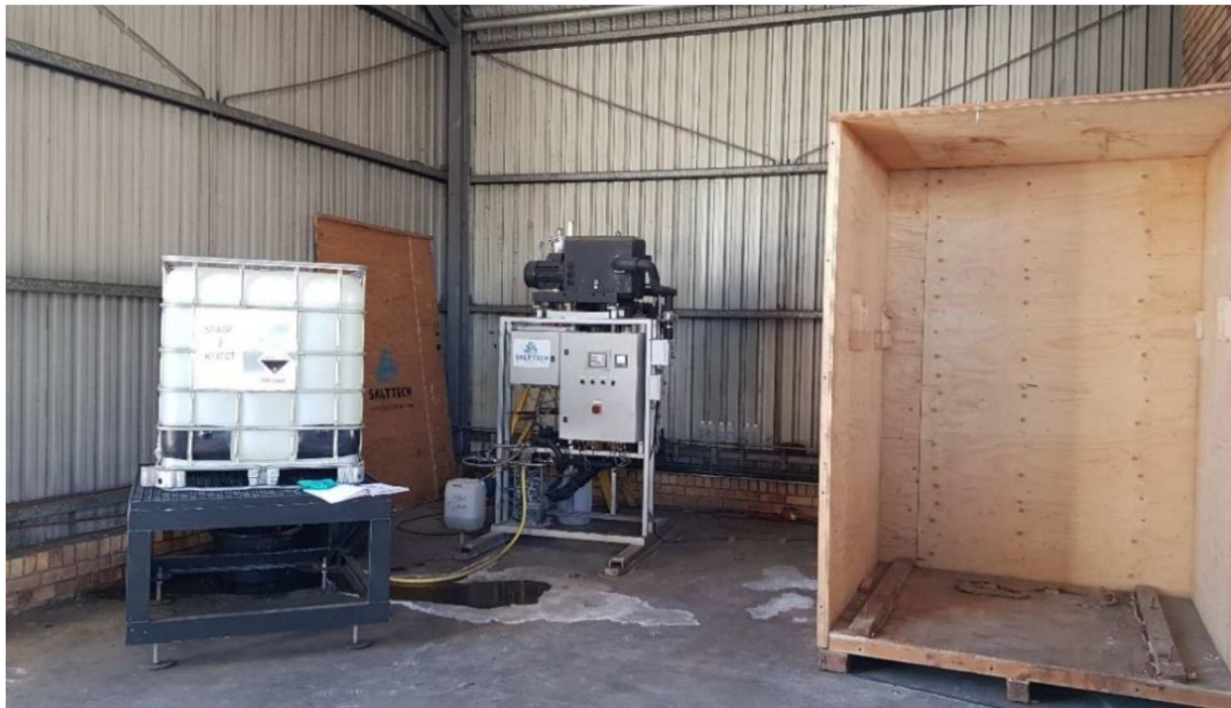
Figure 3.8: EWRP DyVaR pilot plant
