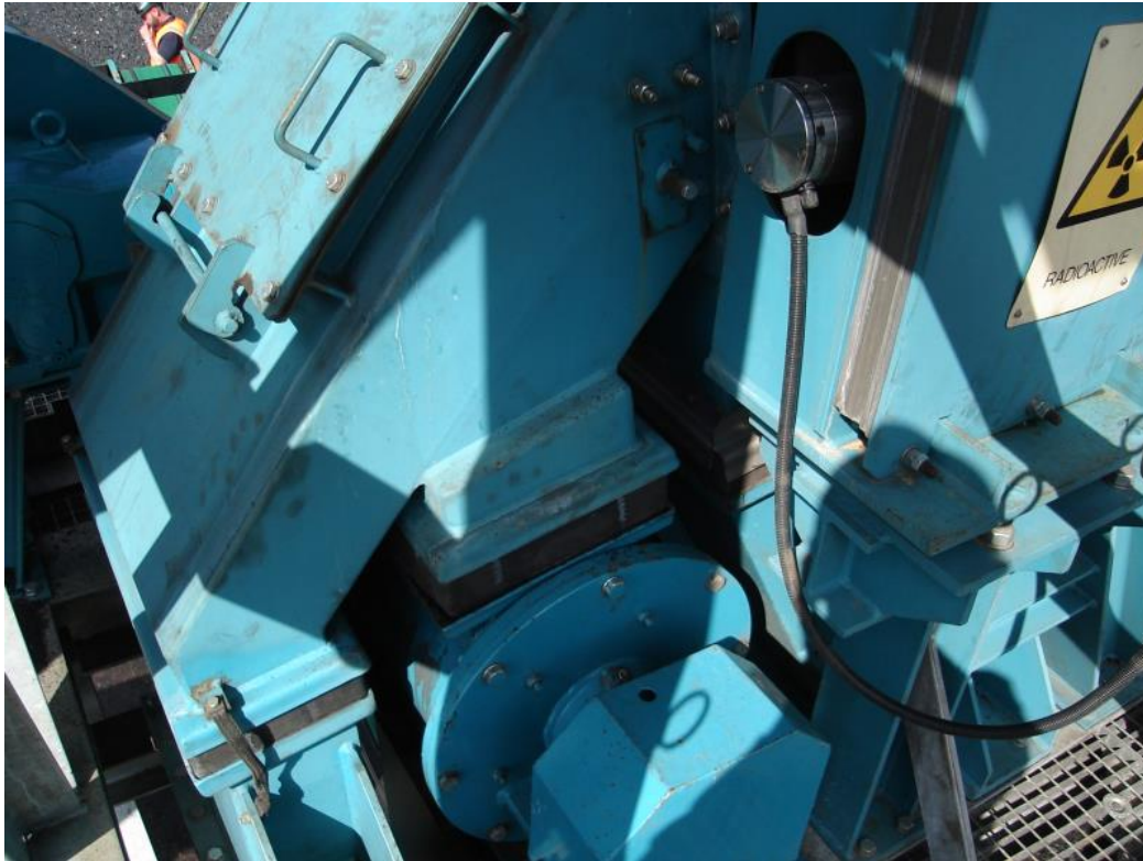
Figure 3: Density gauge and star gate for controlled removal of discard
