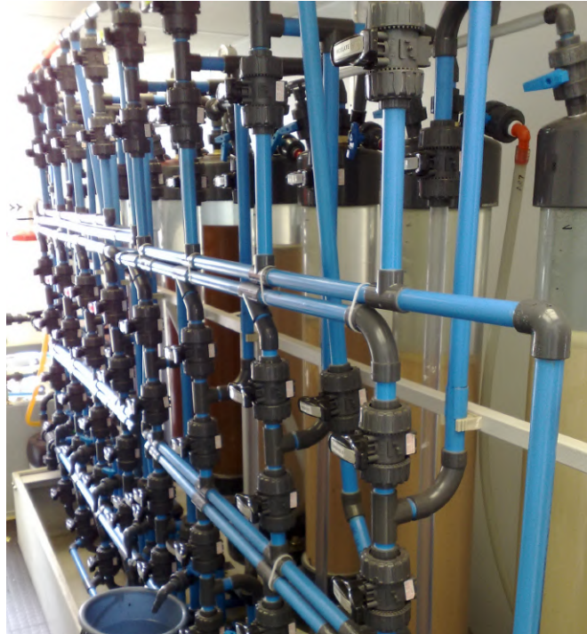
Figure 7. Manifold for operation of the IX portion of the pilot plant
