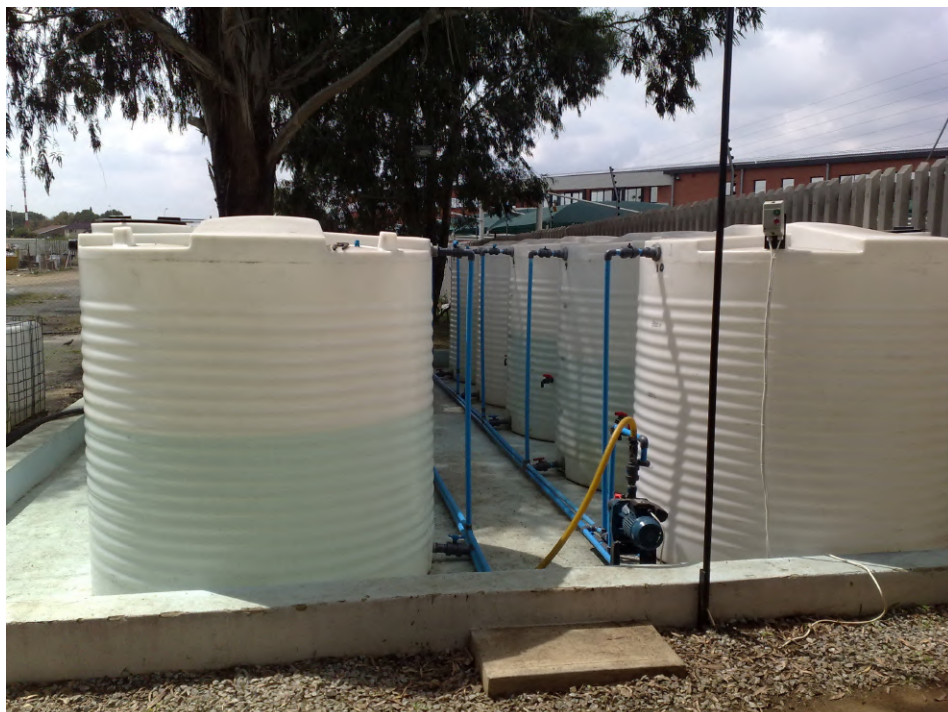
Figure 5. . Tank farm in bunded area at the Earth Boksburg site
