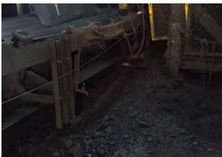
Figure 4: Spillage at transfer point
