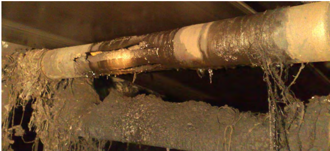
Figure 1: A poorly maintained idler and conveyor system
