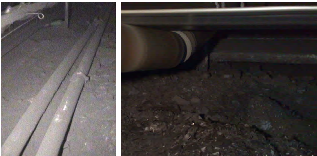
Figure 17: Mine service pipes
