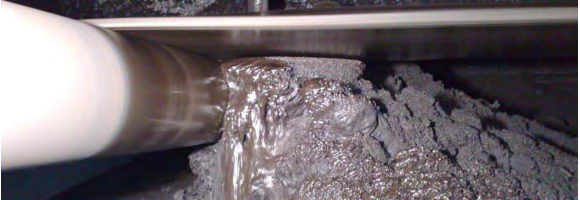
Figure 16: Restricted access below belt
